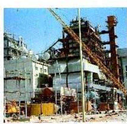
Guddu Power Plant, Pakistan
