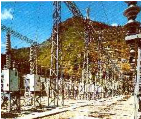
Rio Prado Substation, Colombia
